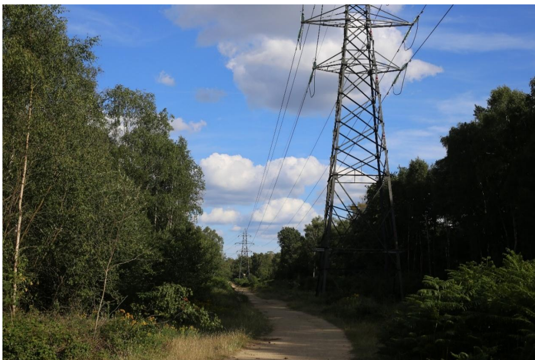
Plate 42: Overhead lines and pylons located within a clearing through dense forest
