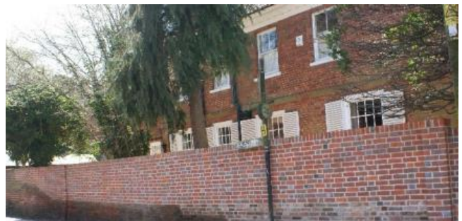
Figure 14 The Cedars, Dippenhall Street; front wall required rebuilding due to vehicular damage
