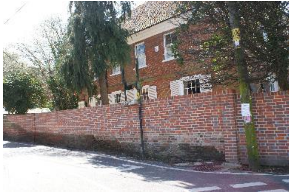
Figure 46 Vehicular damage to The Cedars wall which required rebuilding
